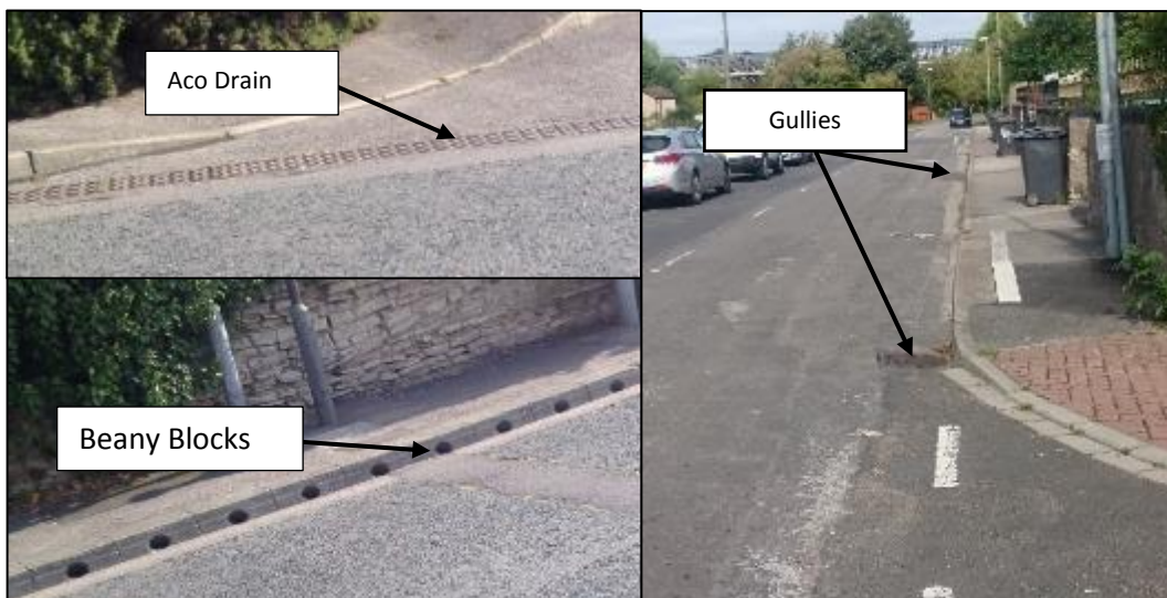
Figure 2.5 Photographs showing Marsh Croft and Low Street drainage systems
