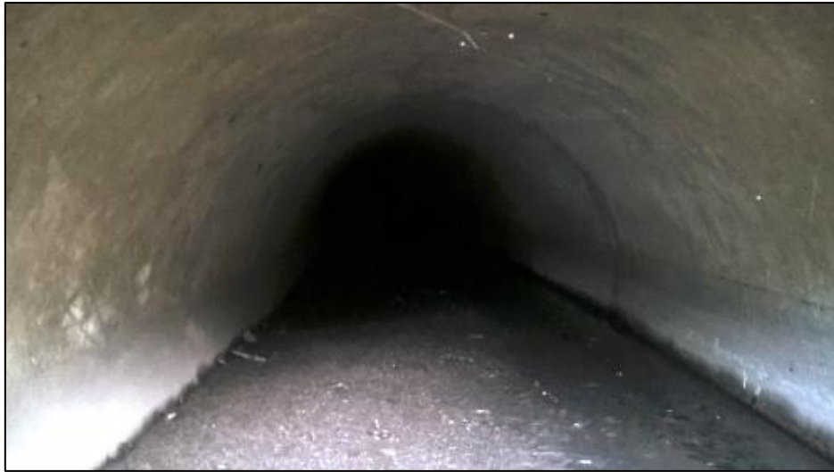
Figure 3.3 Photograph showing silted up culvert under A162
