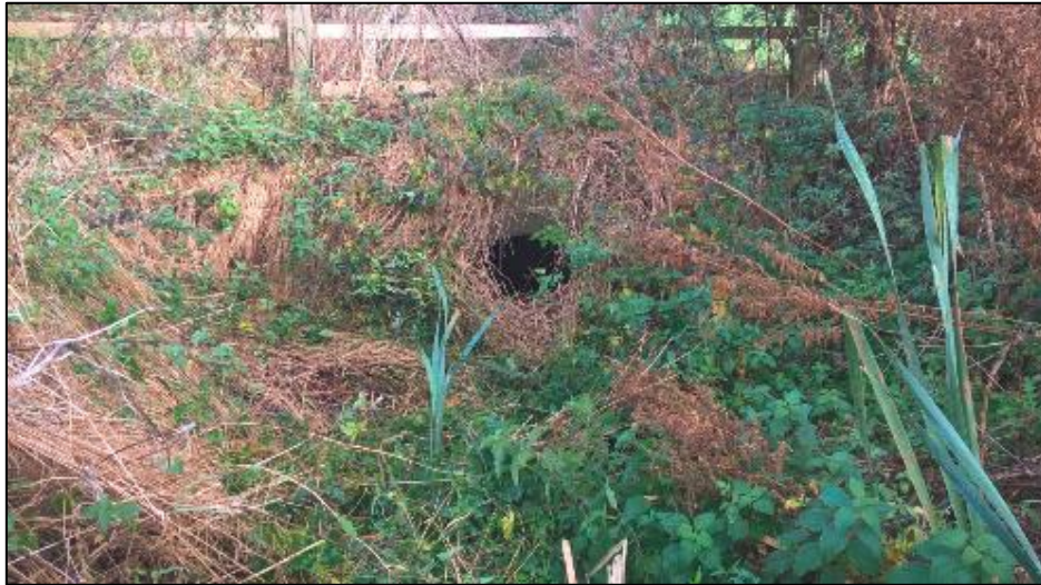
Figure 3.3 Photograph showing vegetation at discharge point of culvert under A162
