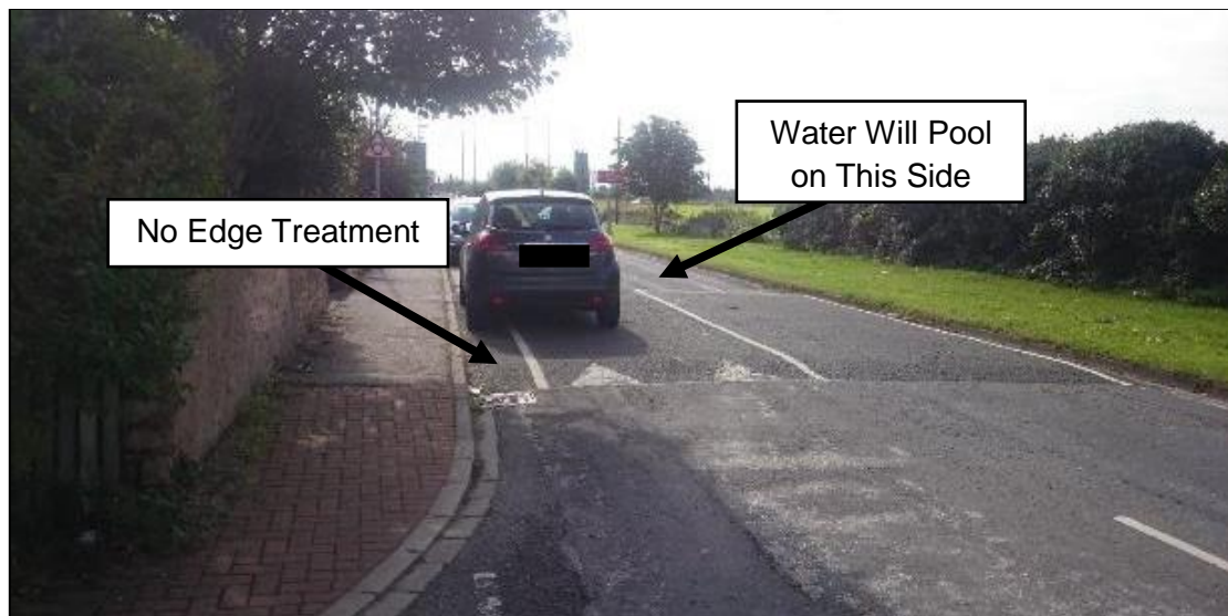
Figure 3.12 Photograph showing lack of edge treatment
